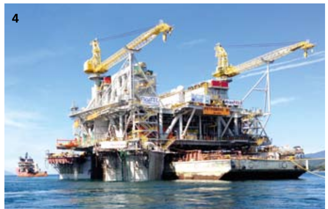
Upon de-ballasting, the hull gradually emerged from the water and connected to the topsides via specially designed receptacles and stab-in cones. Once the topsides had been successfully mated to the hull, the float-over barge was removed from below the topsides, completing the marine mating of the first locally built TLWP for Brazil
