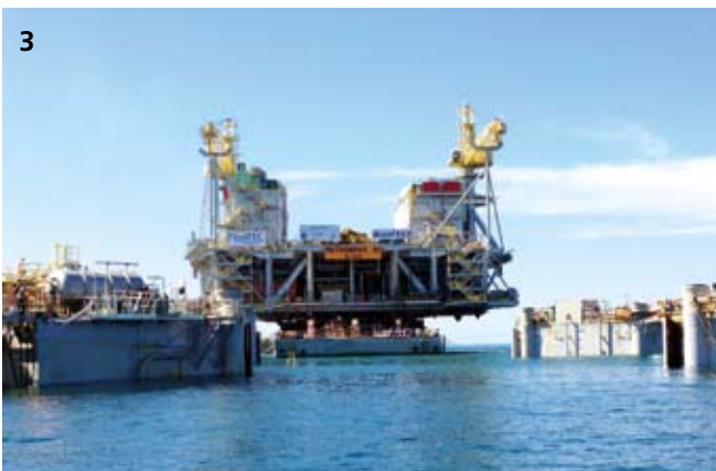
The topsides, which were mounted on a specially built float-over barge, were then towed out and positioned over the submerged four column hull
